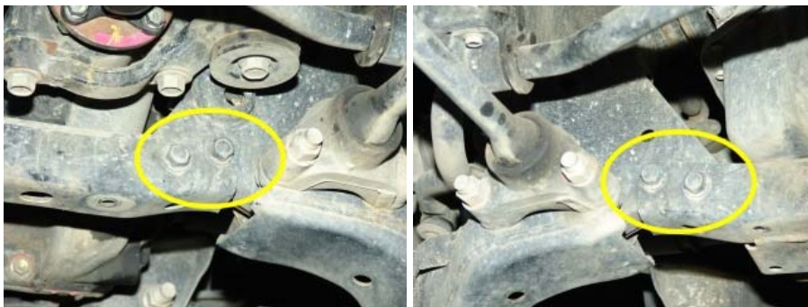
Side bolts of the existing cross member
